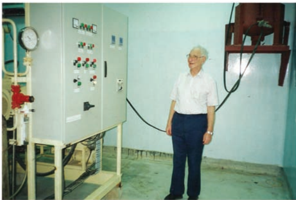
Figure 12: Control panel in place
